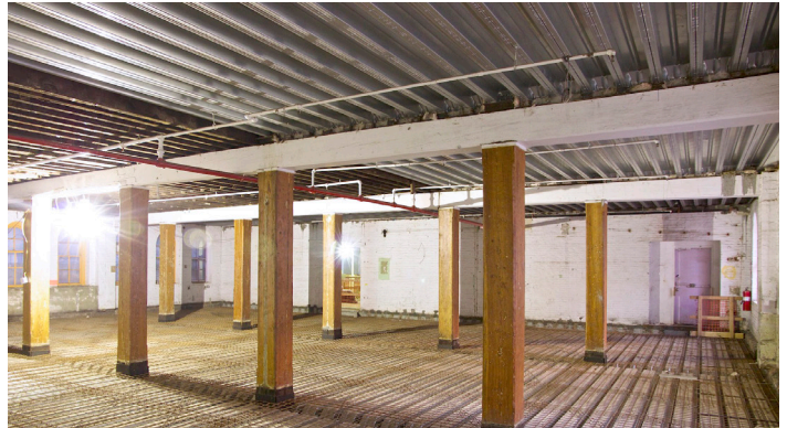
Versa-Floor™ thin-slab composite floors enabled the creation of dramatic ceiling heights at 443 Greenwich Street. Floor-to-ceiling heights were optimized, even with the integration of radiant heating.
