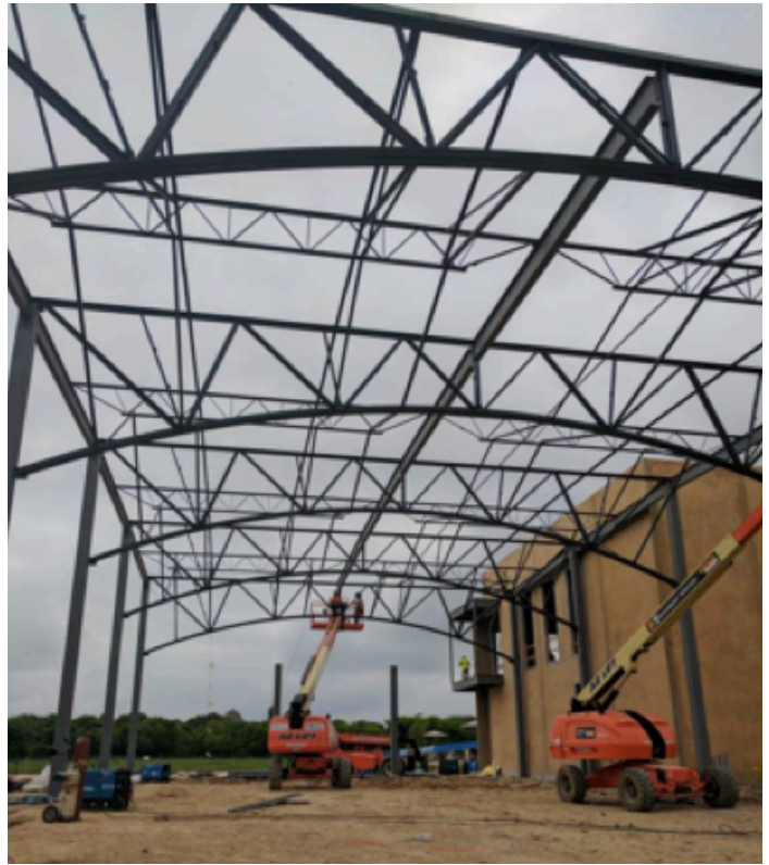
The special joist girders with curved bottom chords designed for the Harvey E. Najim Family YMCA are seen here prior to the installation of the deck above it.
